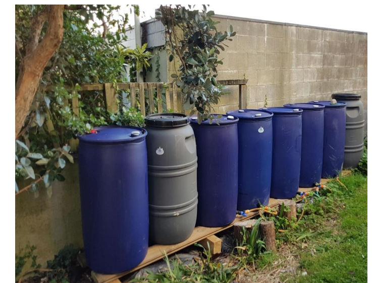
Figure 14 Line up of recycled barrels for rainwater harvesting
